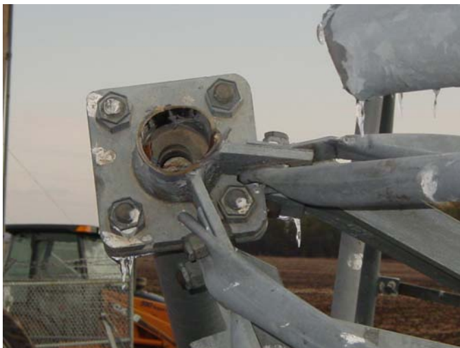
Broken leg from same tower – Normal leg thickness – Nov 2003
