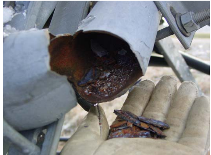
Note leg wall thickness – should be schedule 40. Nov 2003
