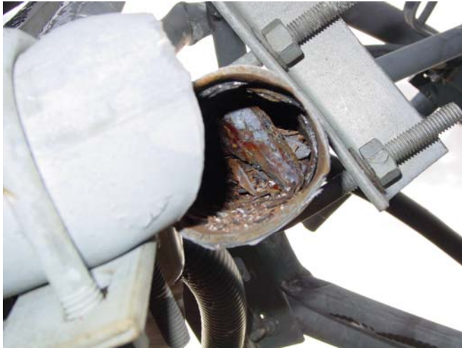
Corrosion inside tower leg – Nov 2003
